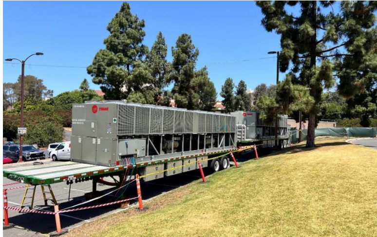
Temporary Cooling and Heating Equipment
