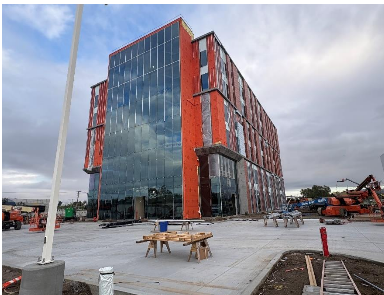
Advantech Campus – Headquarters Building
