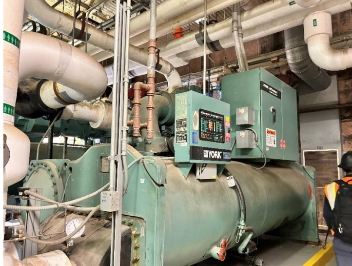
Chiller to be Replaced
