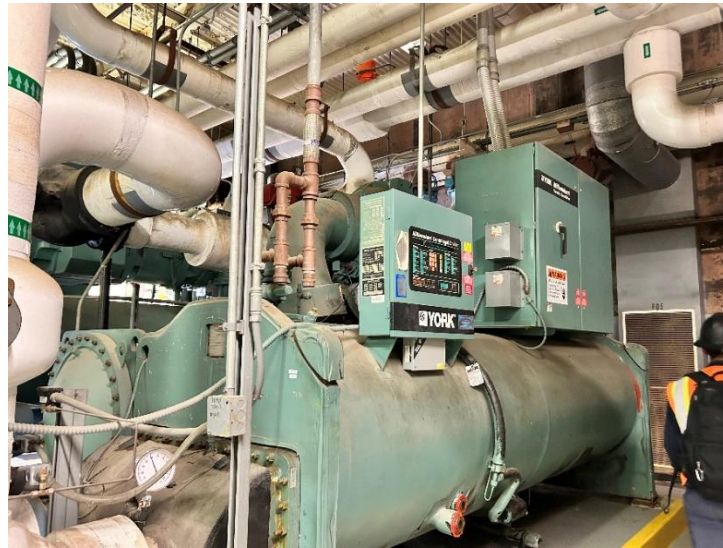
Chiller to be Replaced
