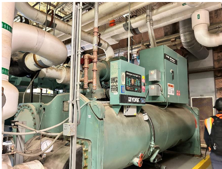
Chiller to be Replaced
