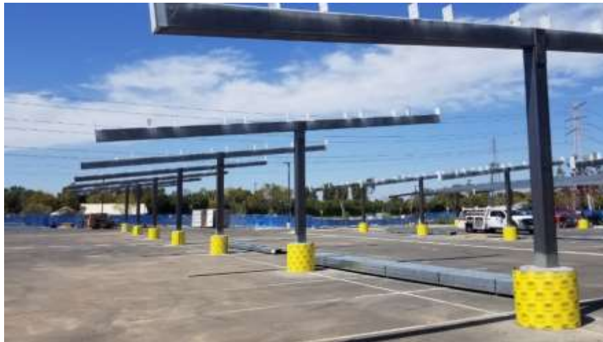
Photovoltaic Structures in Lot 6
