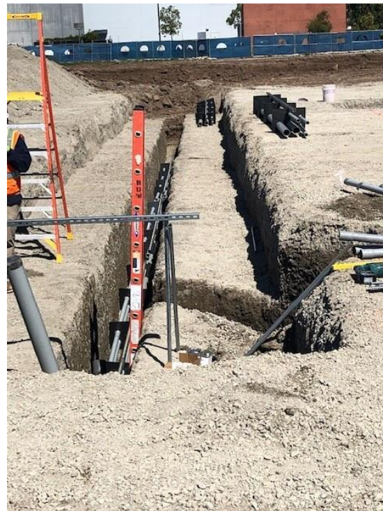
Building B – Underground Electrical Installation
