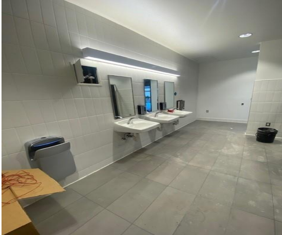
IVC A200 Restroom –Toilet Accessories Installed and Newly Installed Lighting Fixtures Illuminated
