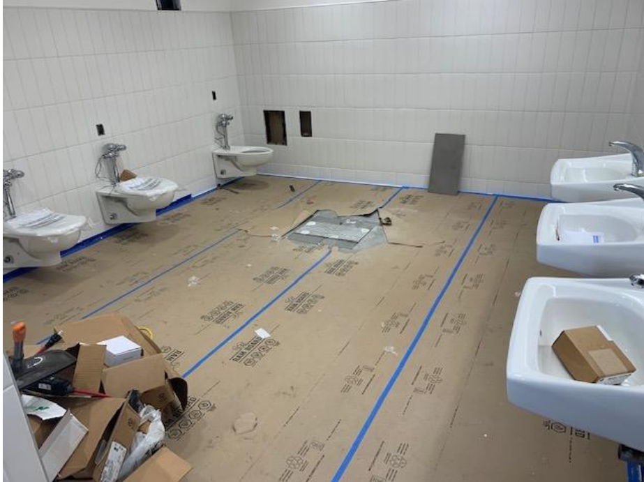
IVC A200 Restroom – Prior to Installation of Access Panels and Remaining Toilet Equipment
