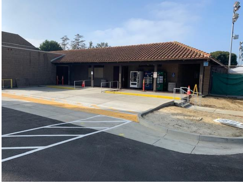
SC Fine Arts PE100 – PE100 Entry Restriped with Newly Installed Galvanized Hand Railing
