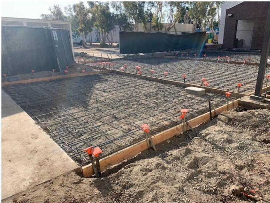
IVC PE Courtyard – Wood Forms and Rebar Installed in Preparation of Final Concrete Pour
