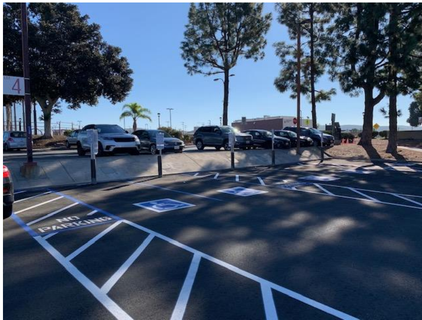
SC Fine Arts PE100 – Asphalt Resurfaced, Restriped, and Handicapped Parking Stall Signage installed
