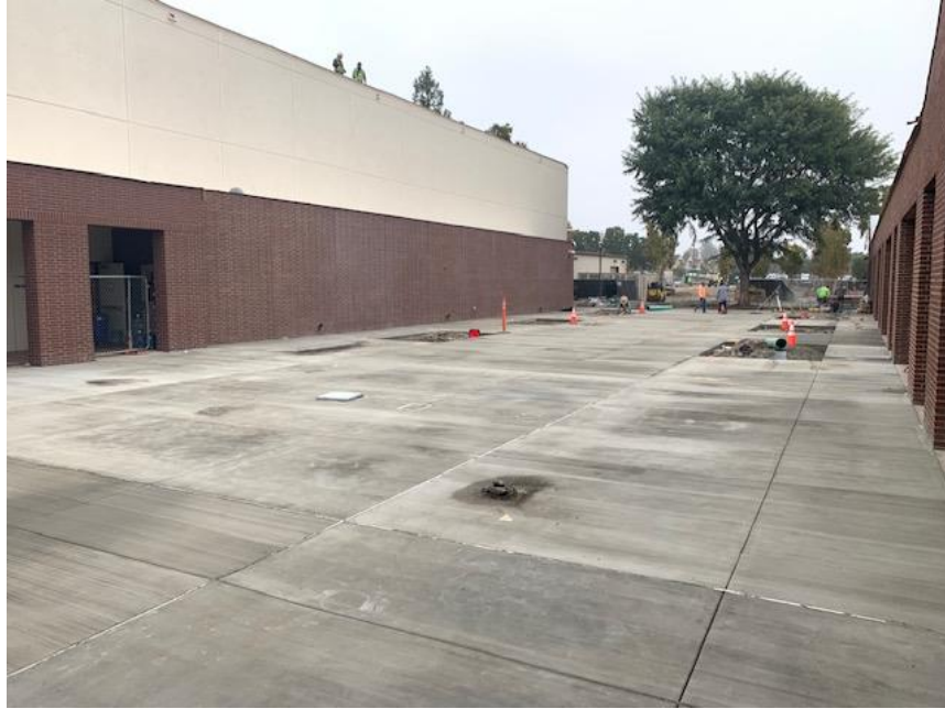
IVC PE Courtyard – New Installation of Concrete Walkway and Concrete Courtyard at PE Building
