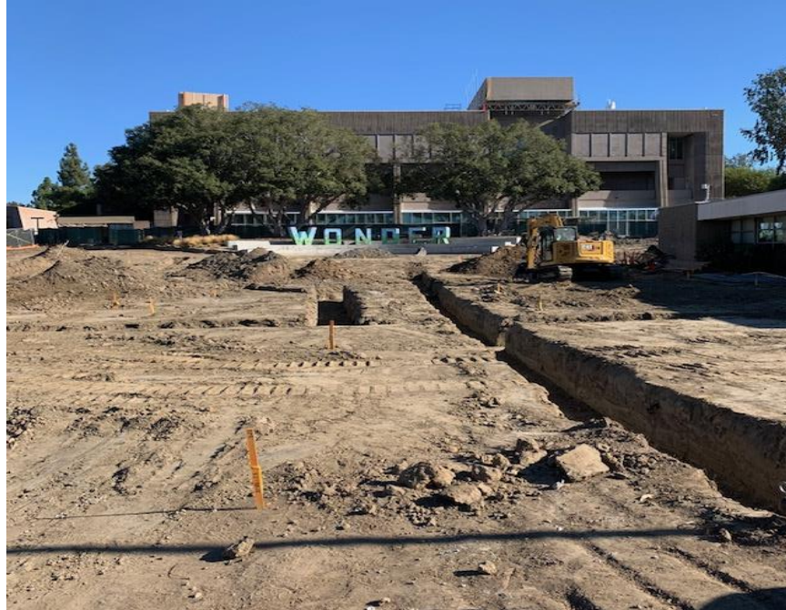
SC Fine Arts Quad Area – Site grading and Fire Line Installation at Saddleback College Fine Arts Quad.
