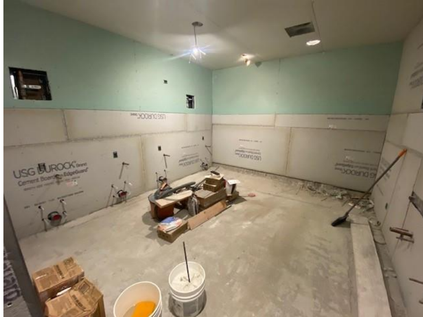
IVC A200 Restroom – Installation of Metal Stud Framing and Drywall at Interior Walls
