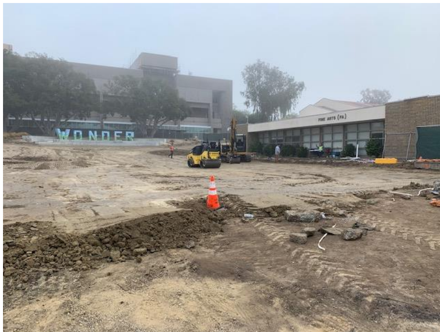
SC Fine Arts Quad Area (Front) – Grading at Saddleback College Fine Arts Quad
