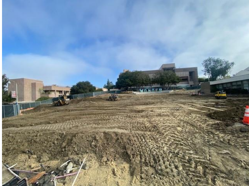
SC Fine Arts Quad Area (Front) – Grading and Removal of Concrete at Saddleback College Fine Arts Quad
