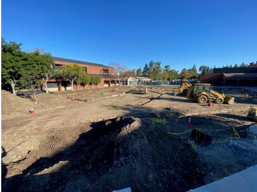
IVC (B Quad) – Grading and Demolition of Site Concrete at Irvine Valley B Quad
