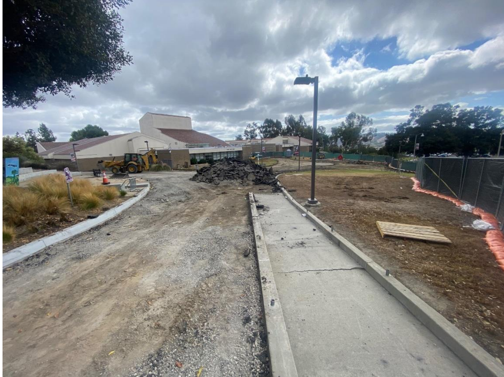
SC Fine Arts Quad Area (Rear) – Grading and Removal of Concrete at Saddleback College Fine Arts Quad
