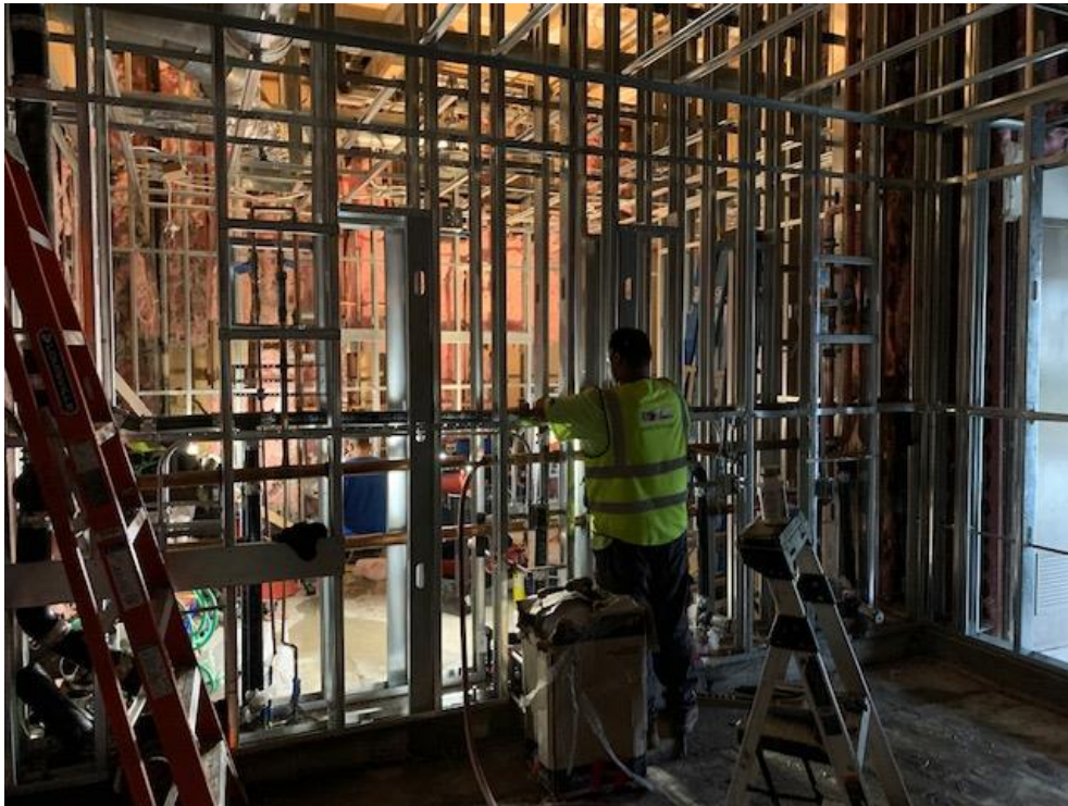
IVC A200 Restroom – Installation of Metal Stud Framing and Plumbing Sanitary Pipe Work
