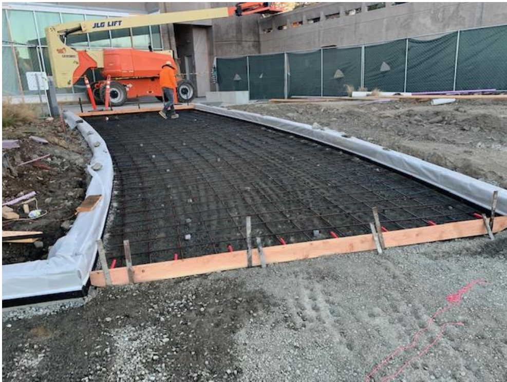
SC Area 5 – Installation of Rebar and Formwork for Concrete Walk Path at Fine Arts Quad
