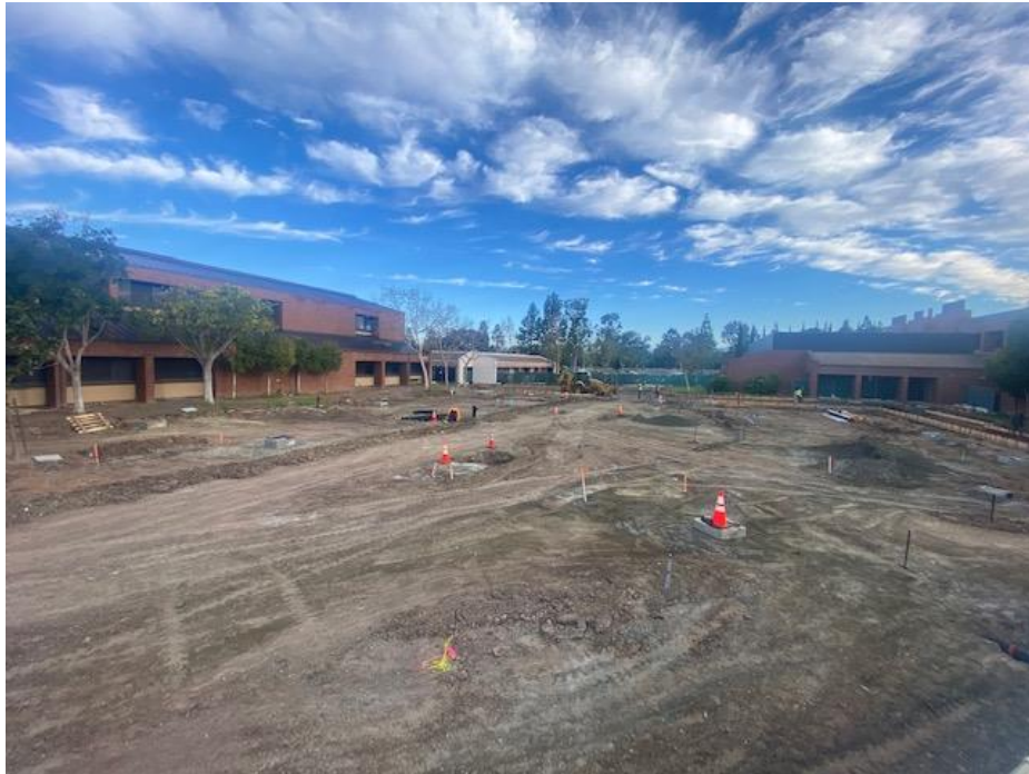
IVC B Quad – Site Overview with Trenches Filled and Formwork Started at Concrete Paving Bands.
