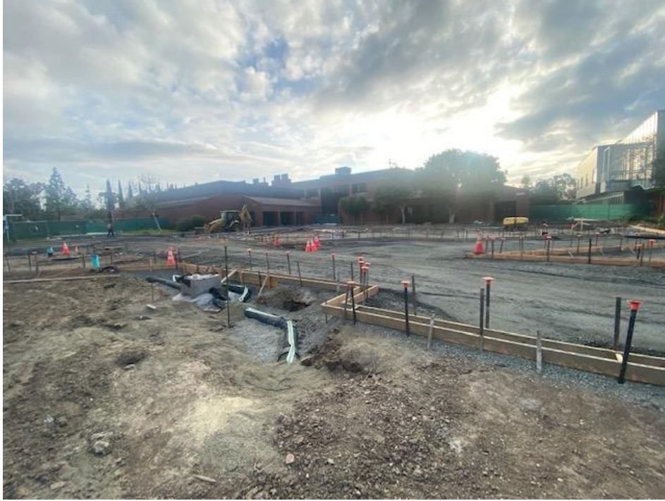
IVC B Quad – Site Overview with Formwork Started at Concrete Paving Bands
