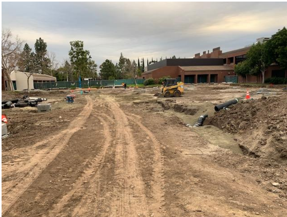
IVC B Quad – Site Overview with New Trenches for Storm System and Storm System Connection
