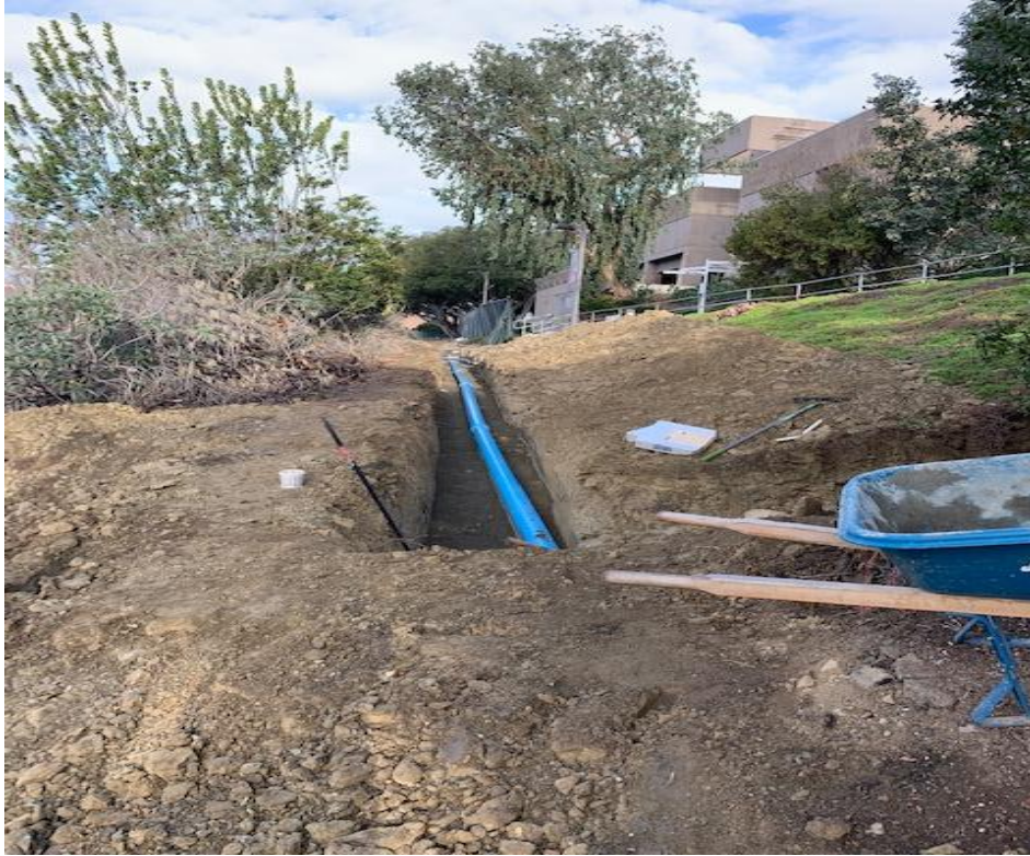
SC Fine Arts Area 5 –Installation of Fire Line Near Fine Arts Quad and Area 6
