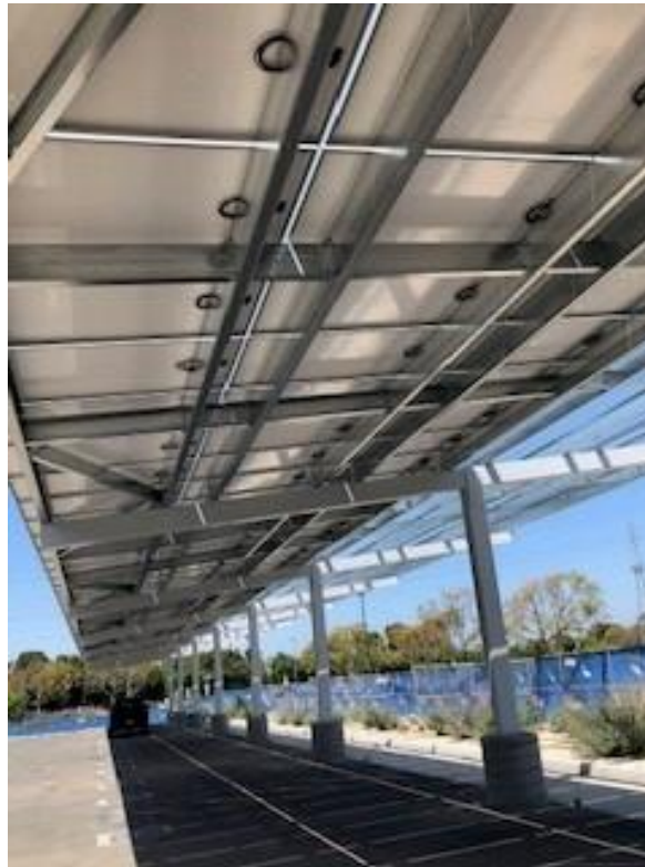
Underside View of Modules
