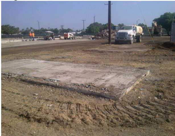
Buildings 505 & 506 – Slab Condition
