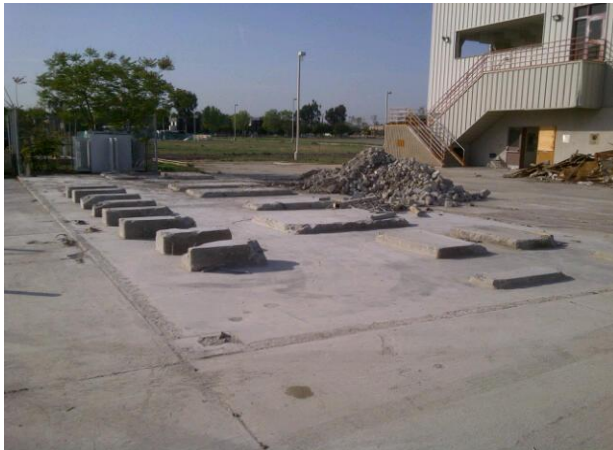
Slab Condition – Building 526
