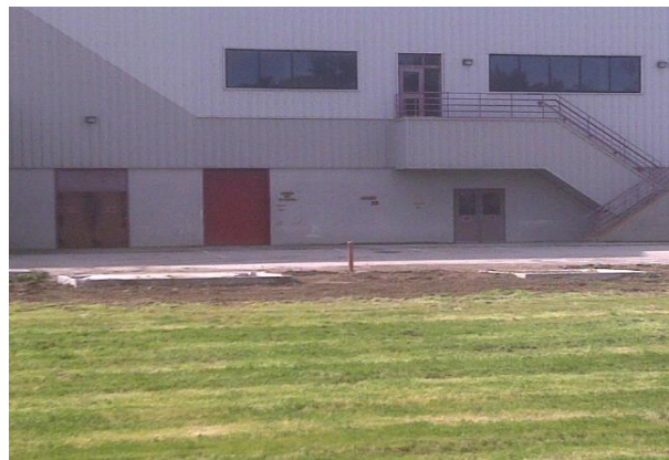
Bldgs. 574 & 602 – Slab condition
